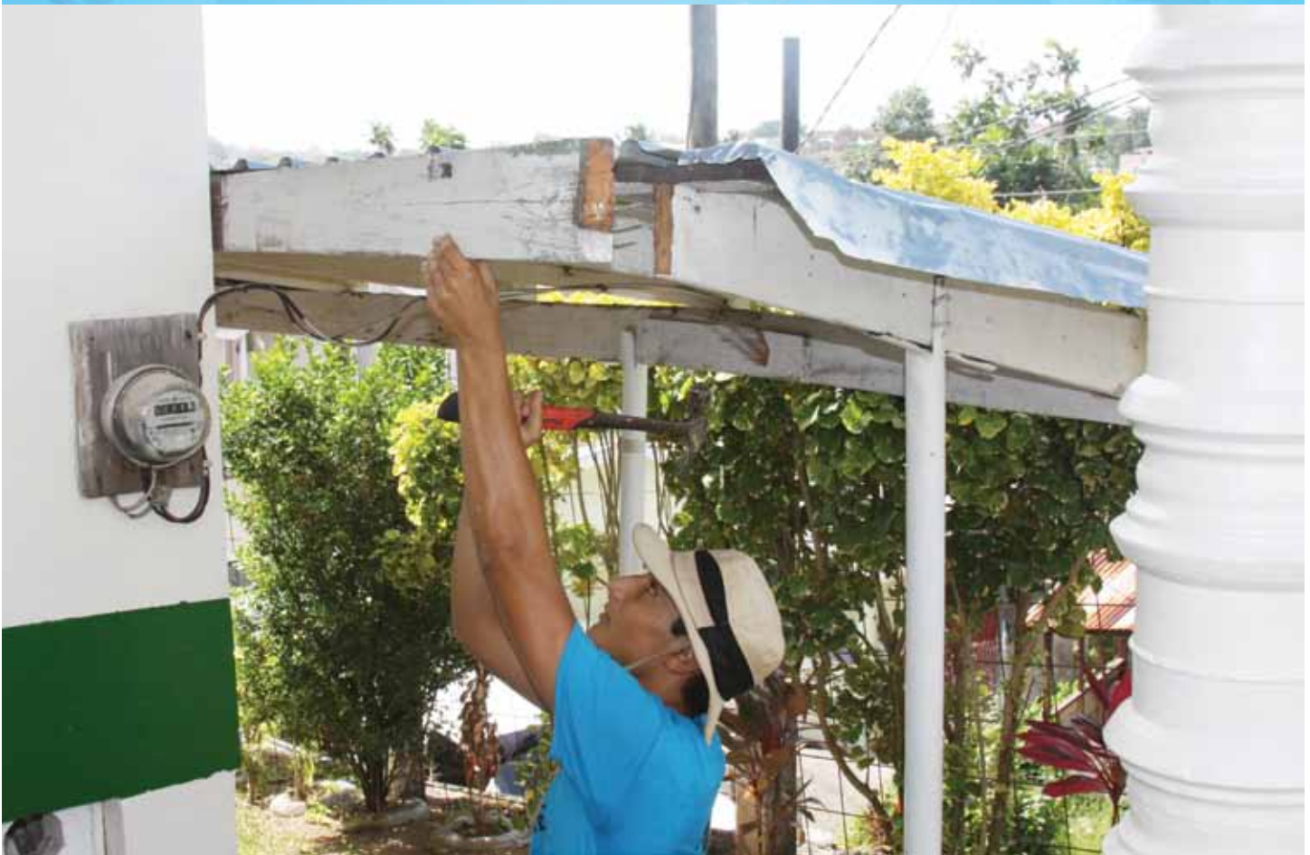
Anthony Dina makes repairs to the roof at Our Lady's Home in St. Lucia while on the diocesan mission trip June 22- June 24.
